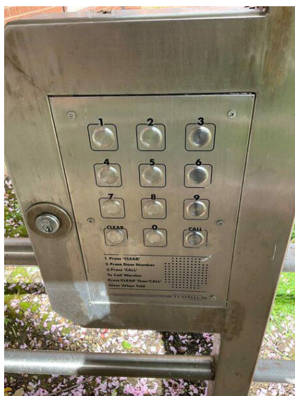
Enlarged key pad on entry to the scheme.
