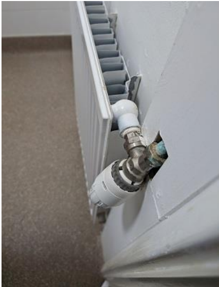
Radiator valve at waist height.
