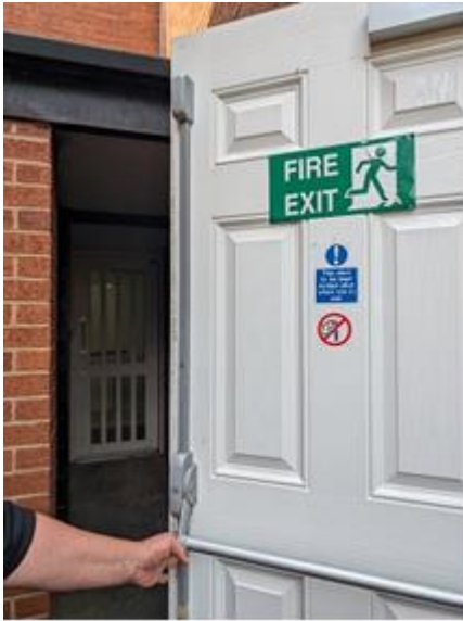
Fire door exit with push handrail.
